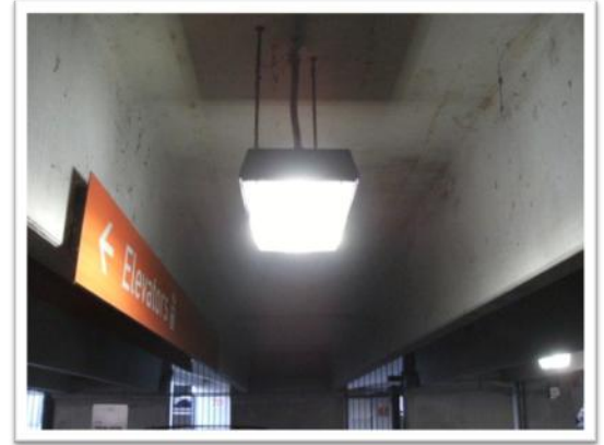
New LED Light fixtures in GBMC garage—ROI slightly over 6 months.
